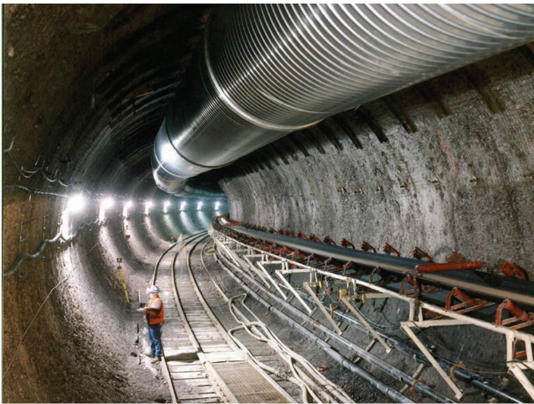
FIGURE 1.1. The underground Exploratory Studies Facility built at Yucca Mountain by the Department of Energy to determine whether the location was suitable as a deep geological repository.
